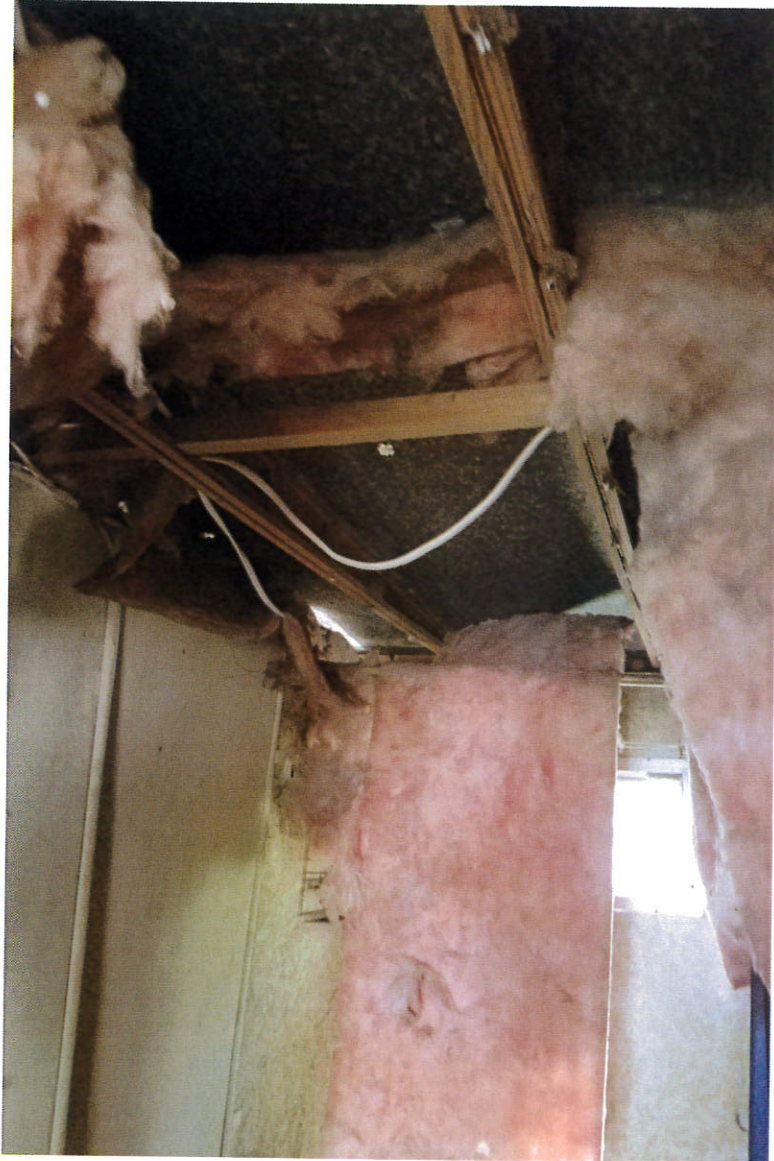
BATH ROOM CEILING
