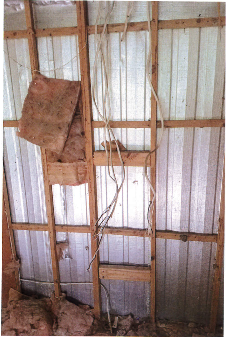
ELECTRICAL PANEL MISSING
