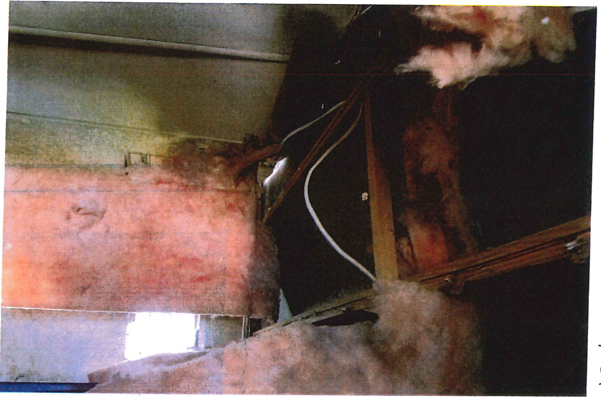
BATH ROOM CEILING
